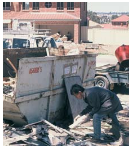
Sorting waste during a waste audit of construction materials at a project-built house (photo David Gardner)
